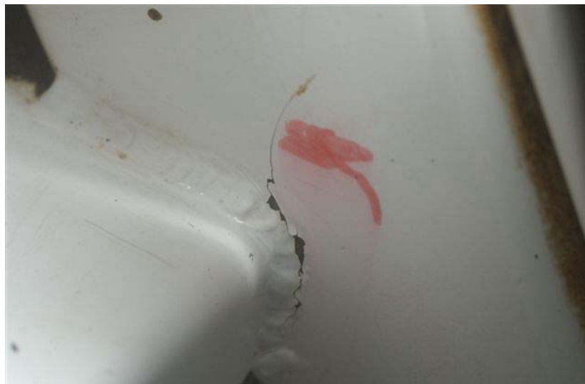
Figure 2. An example of a crack emanating from a welded connection. (Photo. R. Savage)
